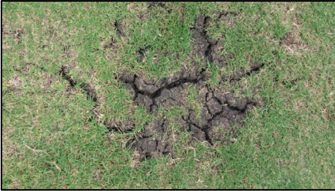
Photo 1. Typical surface cracking in winter on the fairway of a golf course laid out on black swelling clay soils (Akasia, near Pretoria).
